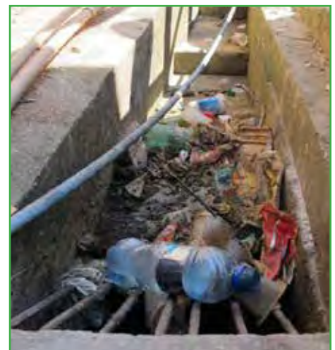
Water carries trash and debris downhill, which can clog storm drains and lead to flooding.
