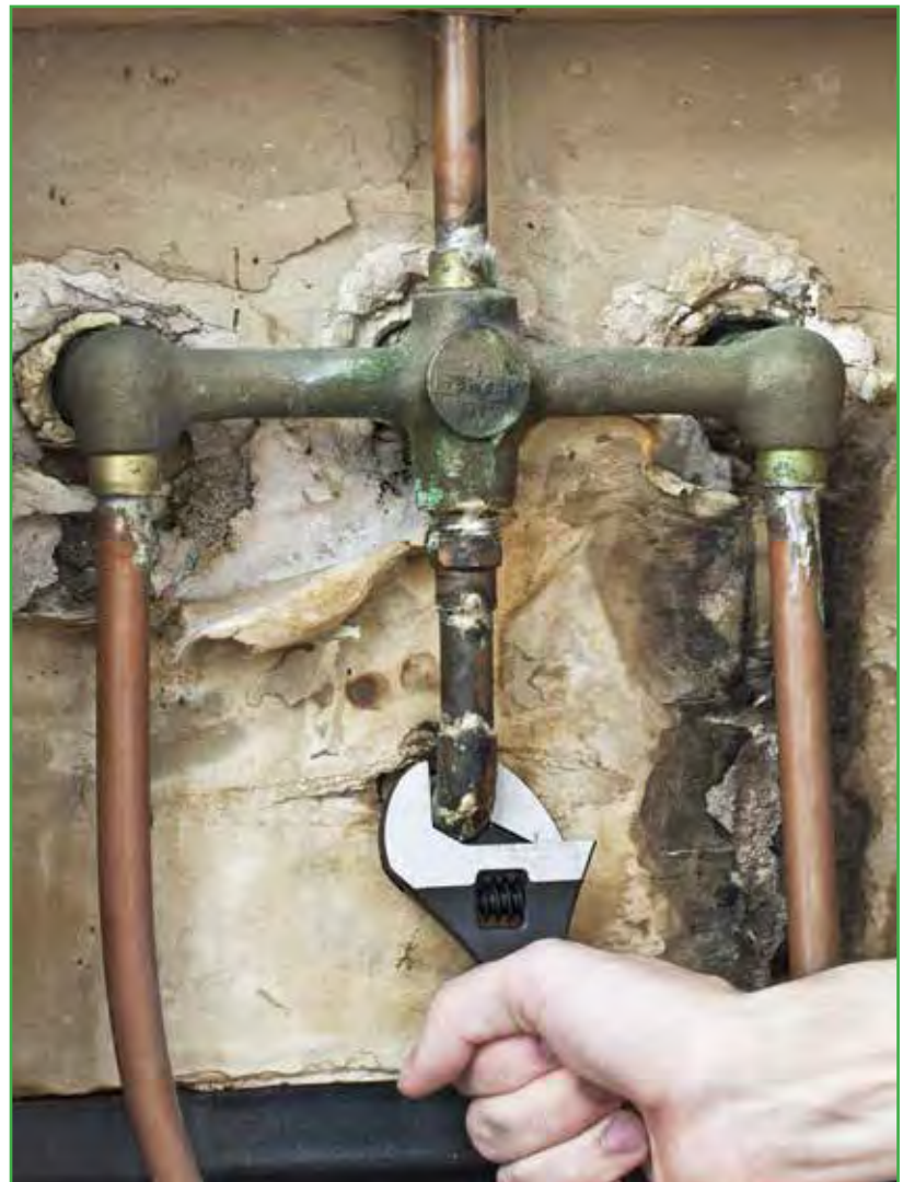
Fixing leaky faucets and toilets helps to conserve water.
